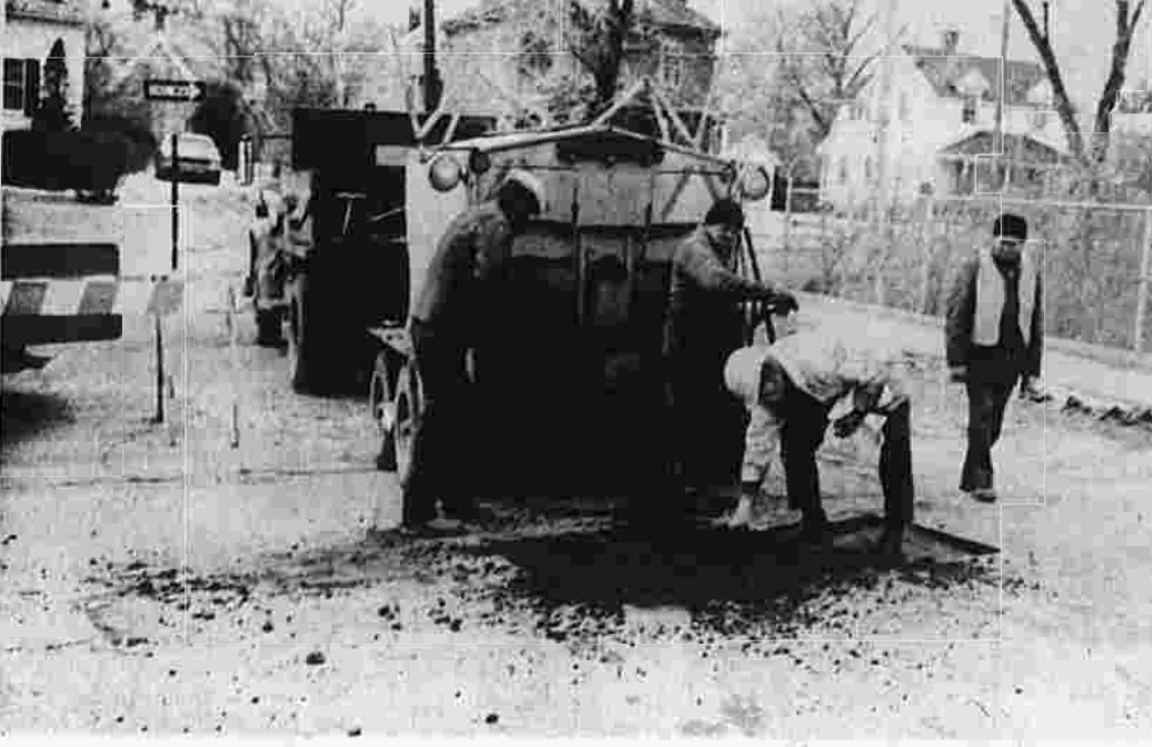
Town workers made temporary repairs to the Park Street Bridge in Manchester Thursday so that the bridge can be used over the weekend. It will be closed early next week for a through inspection of the deck which has shown evidence of corrosion. (Herald photo by Pinto)
